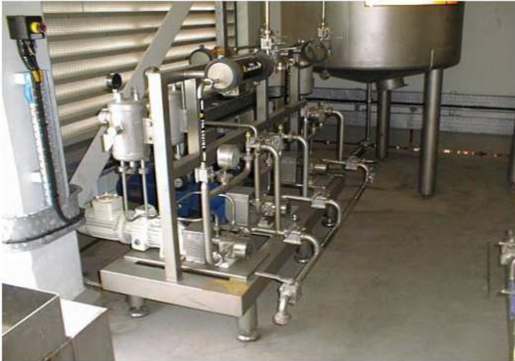
Figure 3: Example of Enzyme Transfer Pump Sets
